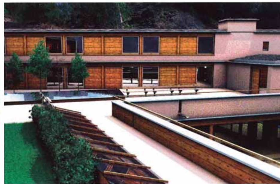
Solid timber decks of mechanically-fixed 6x2s create a warm deck and support the roof terraces above
